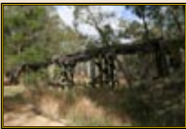
15. MISERY CREEK BRIDGE Opened with great celebration in 1906. The 70ft long bridge was once the main crossing of Mount Misery Creek.
